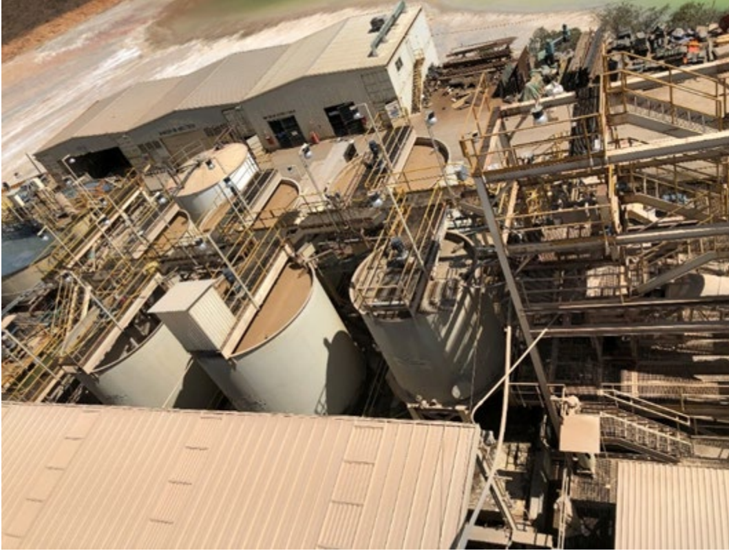
Figure 14-87: Agitated Leach Circuit of the DDGM Processing Facility.
