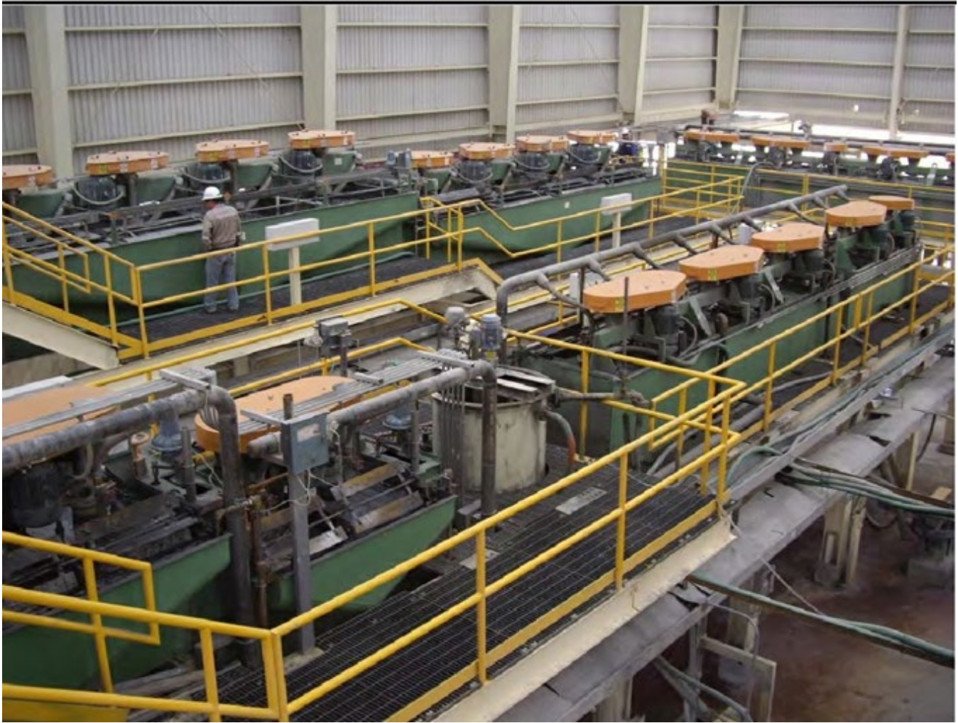
Figure 14.4 Banks of Flotation Cells at the DDGM Processing Facility
