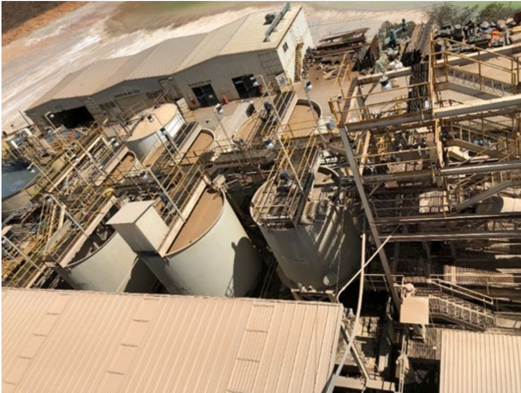
Figure 14.5 Agitated Leach Circuit of the DDGM Processing Facility
